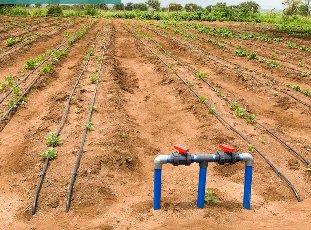
New irrigation system at Naitolia Primary School garden.
